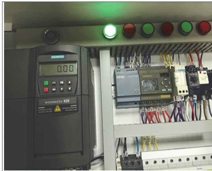
Figure 4. Green indicator 1 “MAIN POWER PRESENTED”
