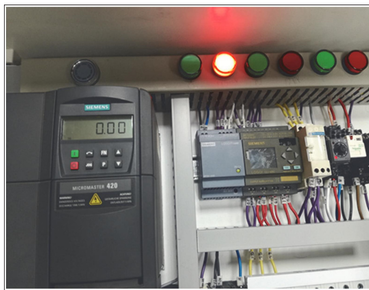
Figure 5. Red indicator 2-alarm “ NO MAIN POWER”
