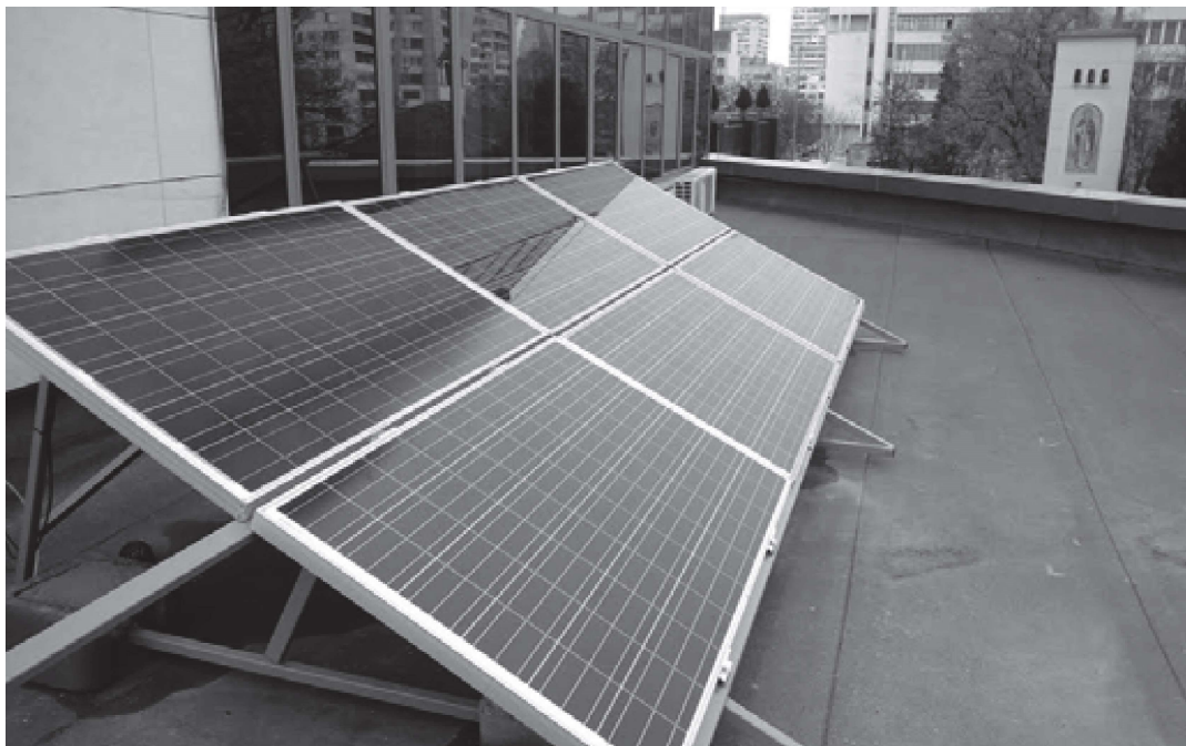
Figure 3. PV-central on the roof of BFU
